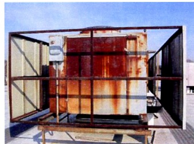
High School Roof Top Unit
